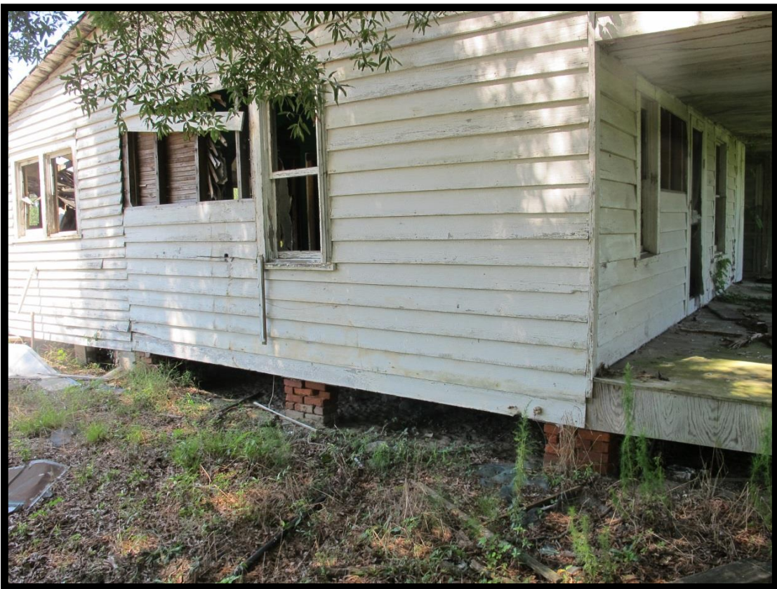
Figure 28: Redmond H. White House (# 012), Detail of East Gable End Showing Brick Pier Foundation.
